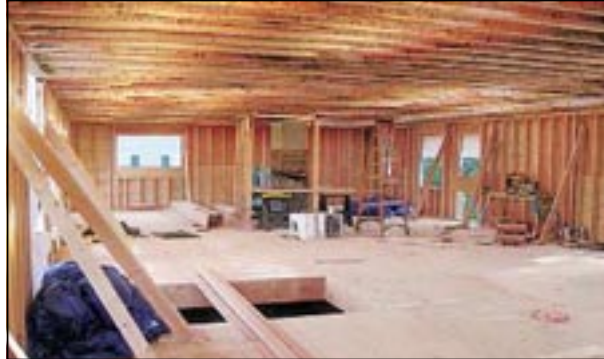
Interior of the North Haledon project, which doubled the size of the home.
